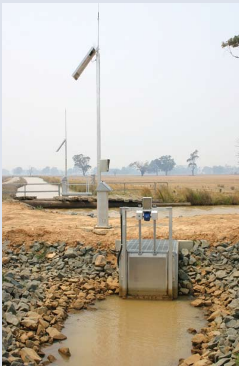
Under the National Framework for Non-Urban Water Metering, new meters such as this one, correctly installed, will improve water accounting nation-wide.
